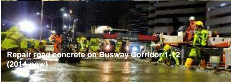
Repair road concrete on several toll road such as : Jagorawi, CTC, Japek, Sumo, Surgem (2012 -now)
