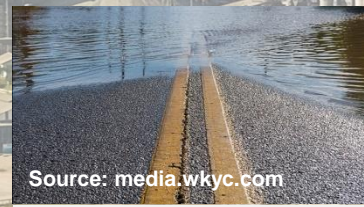
Vulnerable To Flooding
