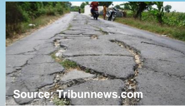
Poor Pavement Structure
