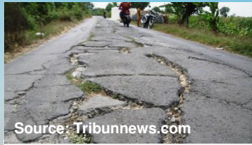
Poor Pavement Structure
