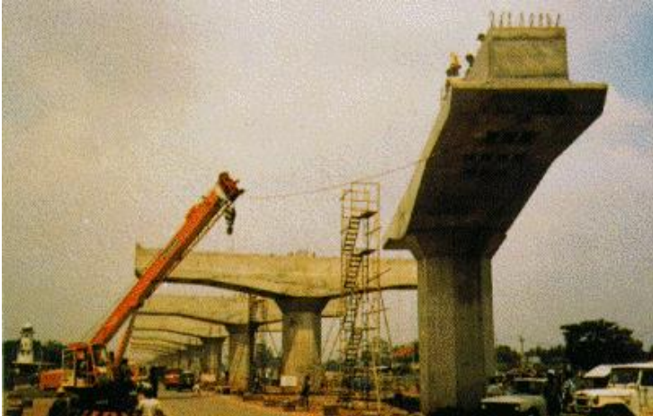
Sosrobahu technology to allow traffic flow during elevated structure construction (will be used in Jakarta – Cikampek Elevated Toll Road)
